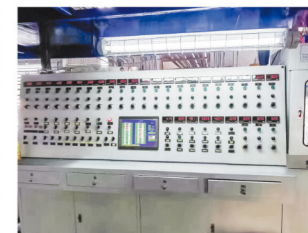
控制柜 Controlling box
